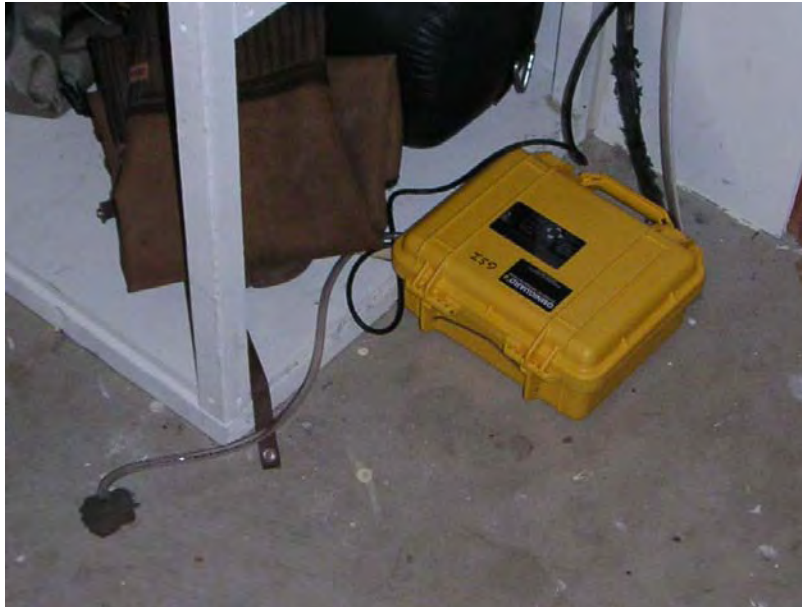
Figure 3.5.7.3 Pressure Transducer Installed to Measure Cross-Foundation Pressure Gradient.
