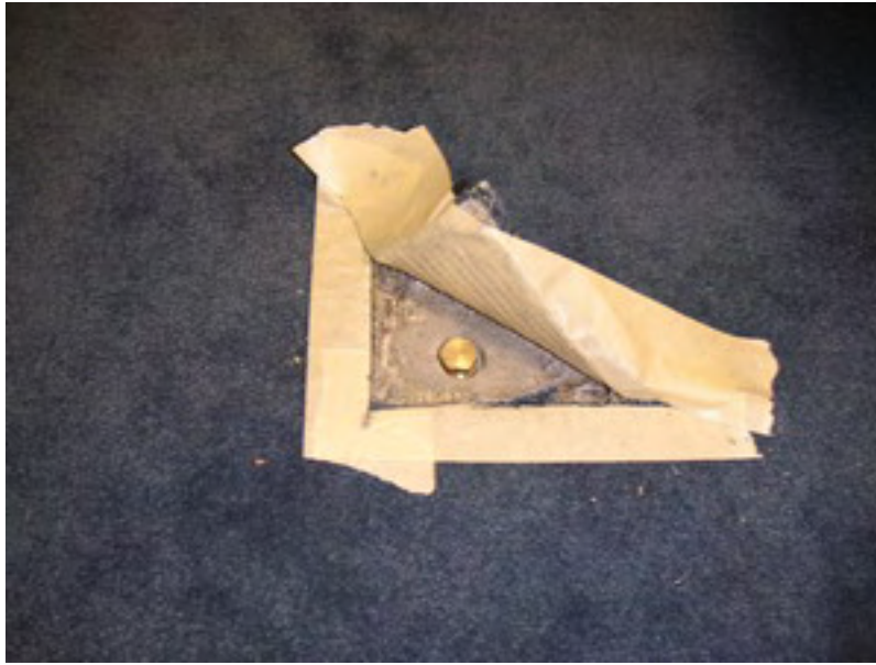
Figure 3.5.1.3 Sub-Slab Sample Port.
